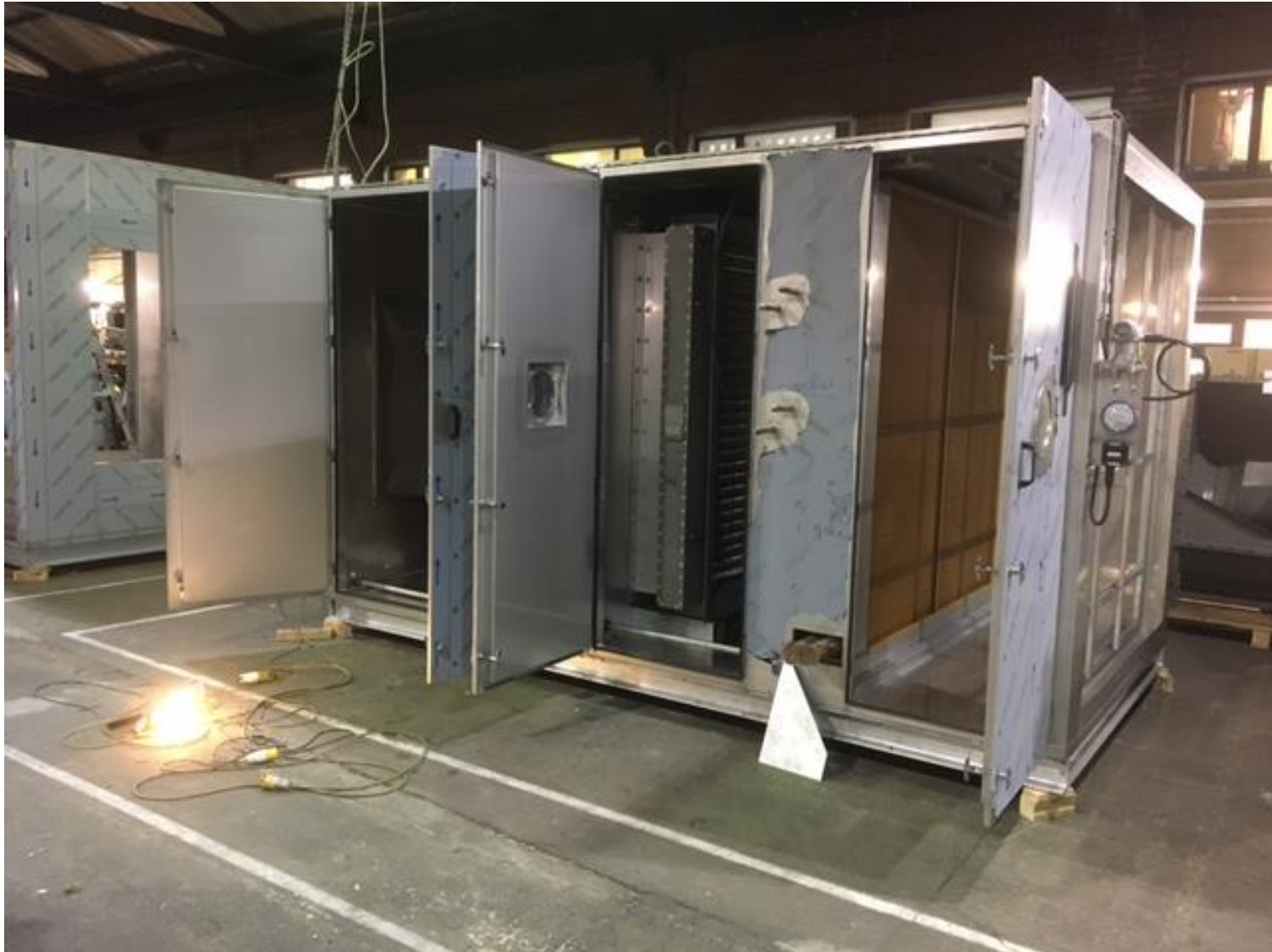
AHU showing cooling coil (Heresite coated) and Heating section
